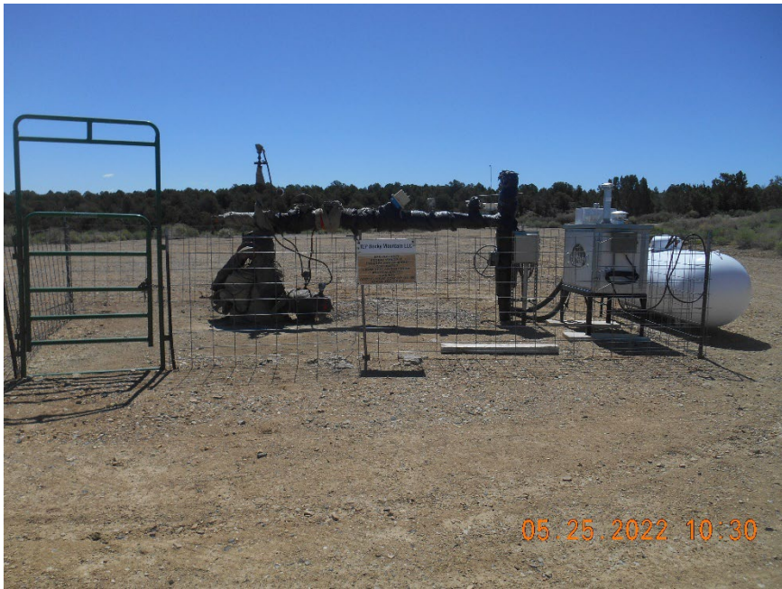
Injection wellhead & line heater
