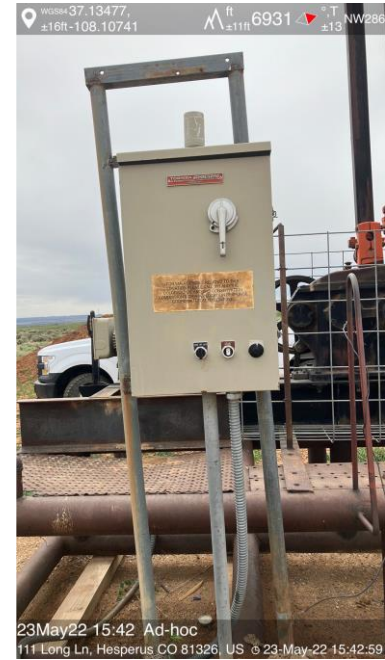
IMG 06 Electric Prime Mover
