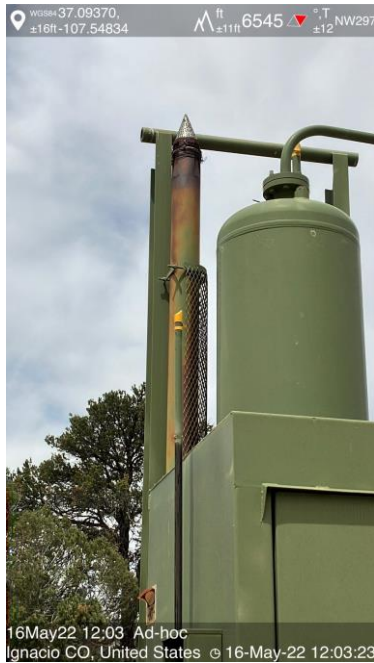
IMG 07 Separator vent stack properly screened
