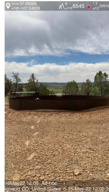
IMG 08 Produced water tank metal berm
