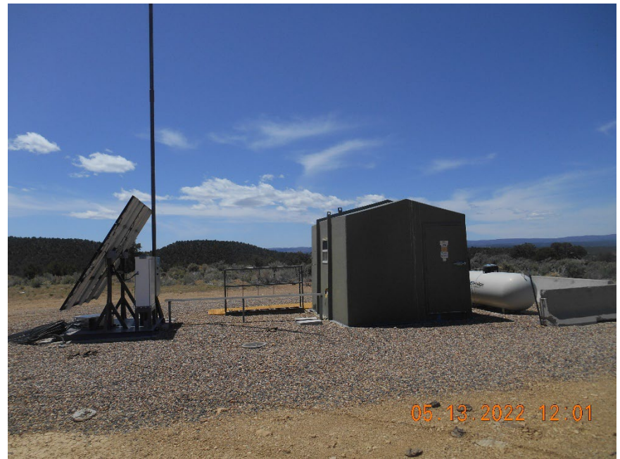
Injection wellhead inside housing
