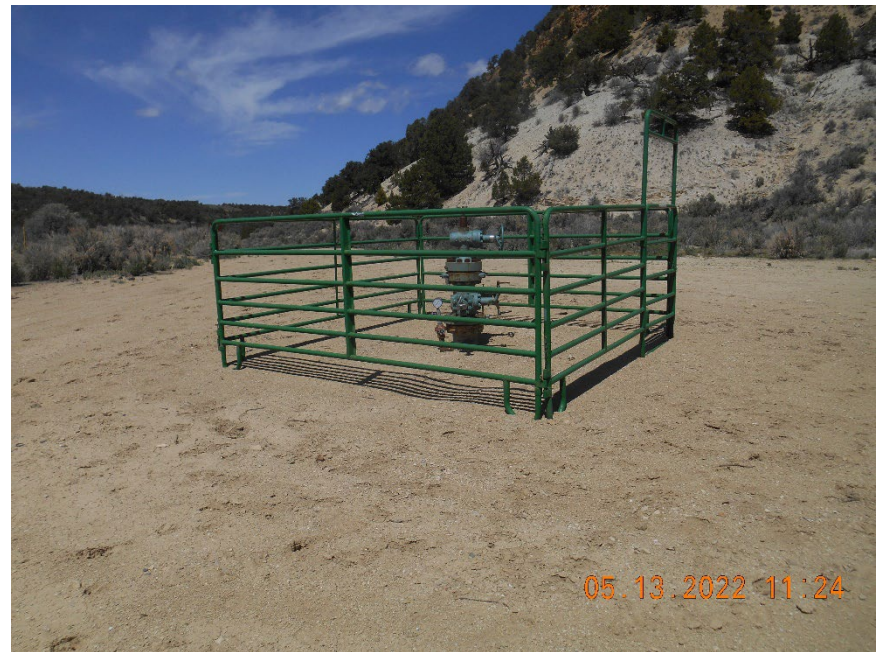
Injection wellhead with fence. Temporarily Abandoned
