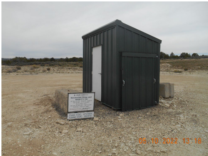
Injection wellhead inside housing.
