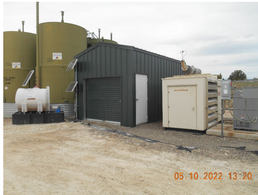
Pump Housing. Chemical injector with secondary containment.
