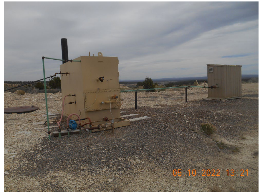
Separator and Meter housing
