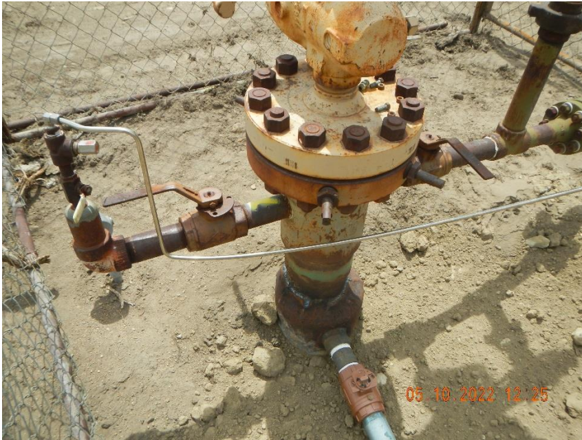
Surface casing has been weld to production casing to create a braden head.
