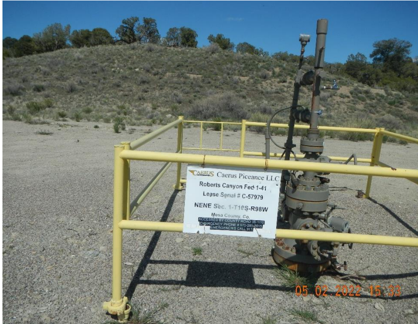
No api # on well sign.
