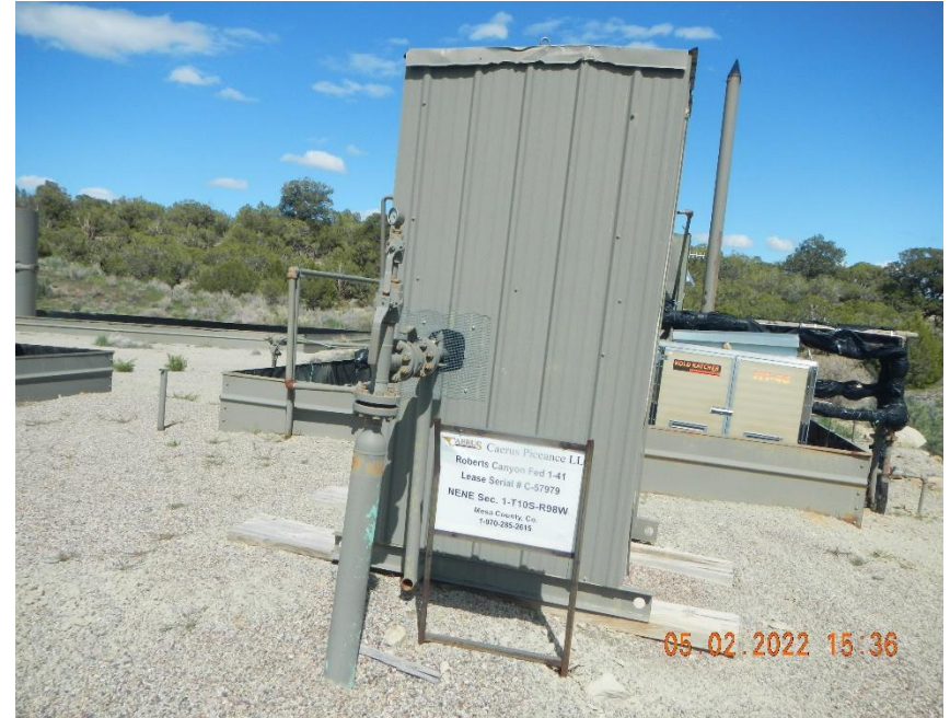
Battery sign at meter shed. Sign missing api # and nearest public road.
