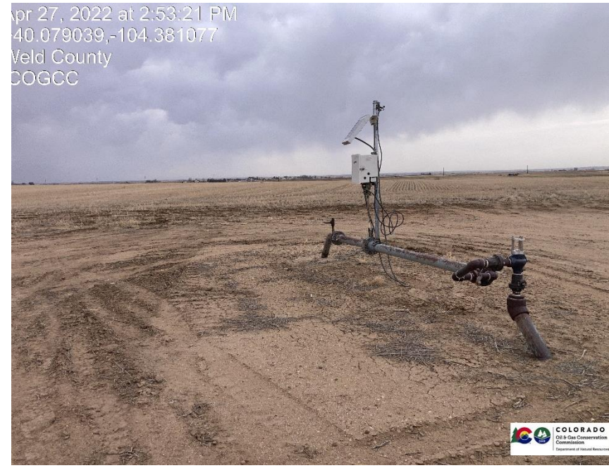
Pic 2 gas meter run
