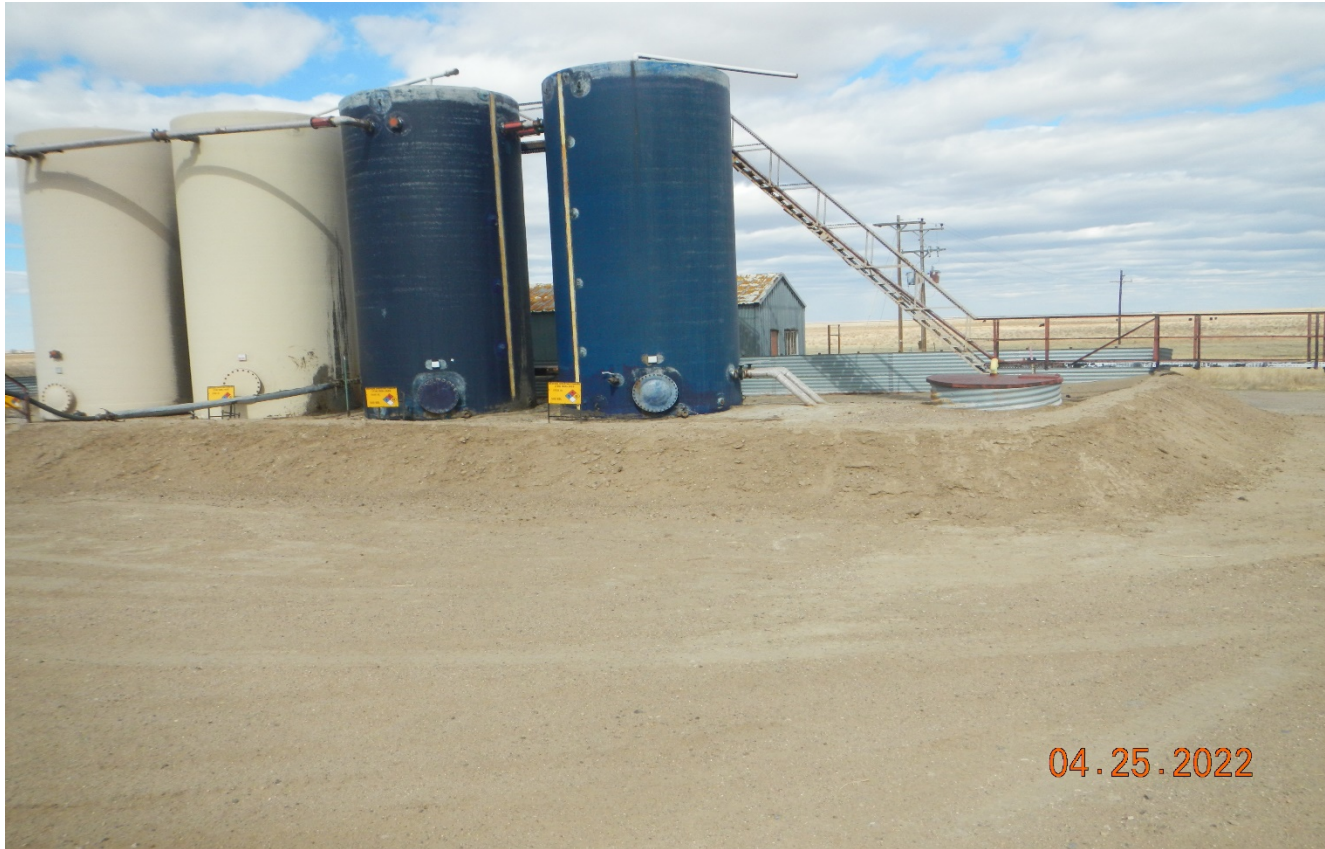
Photo 3. Facing northeast toward the tank battery. The berm around the battery has been repaired.
