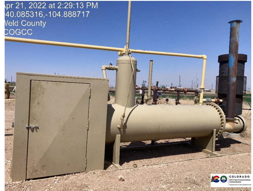
Pic 4 Separator, ECD
