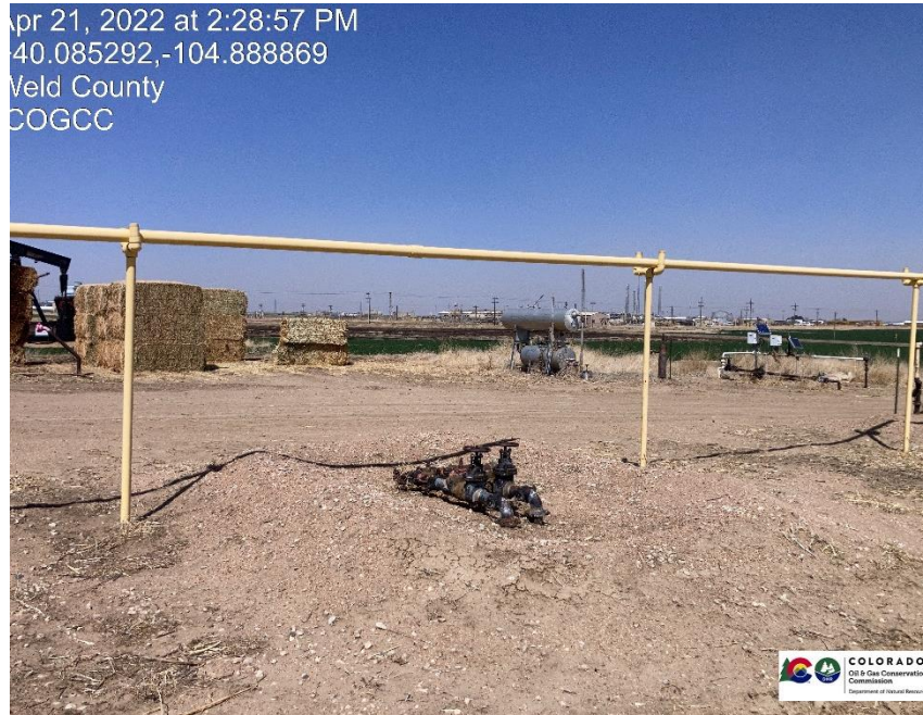
Pic 3 separators, manifold
