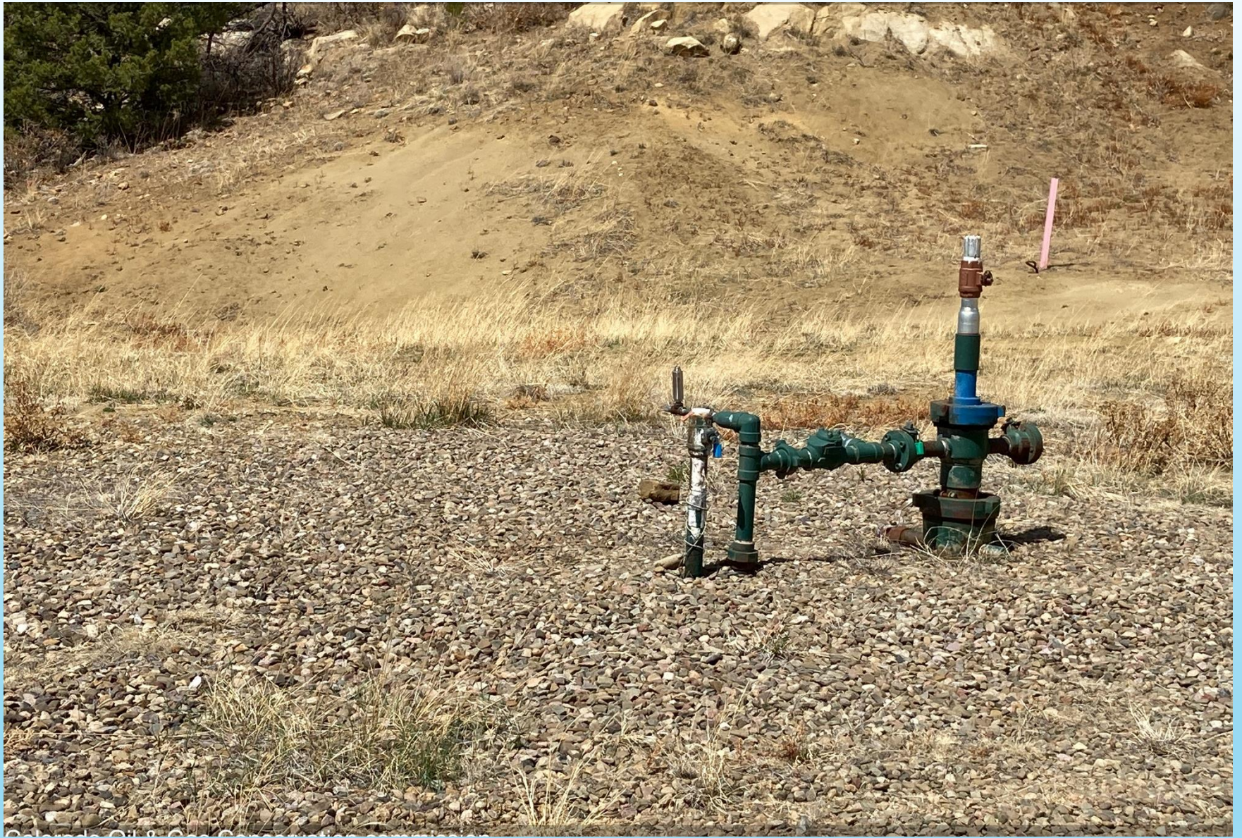
PHOTO 3: WELLHEAD AND EQUIPMENT
