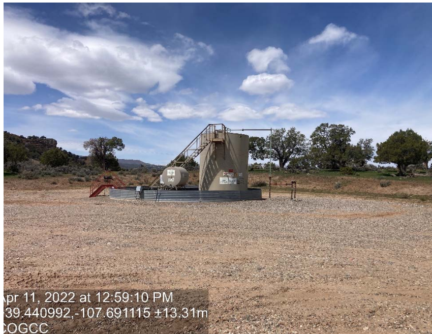
Location/ lack of battery signage
