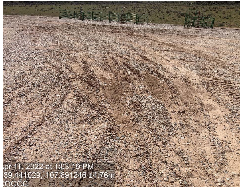
Some areas of lack of stabilization/compaction
