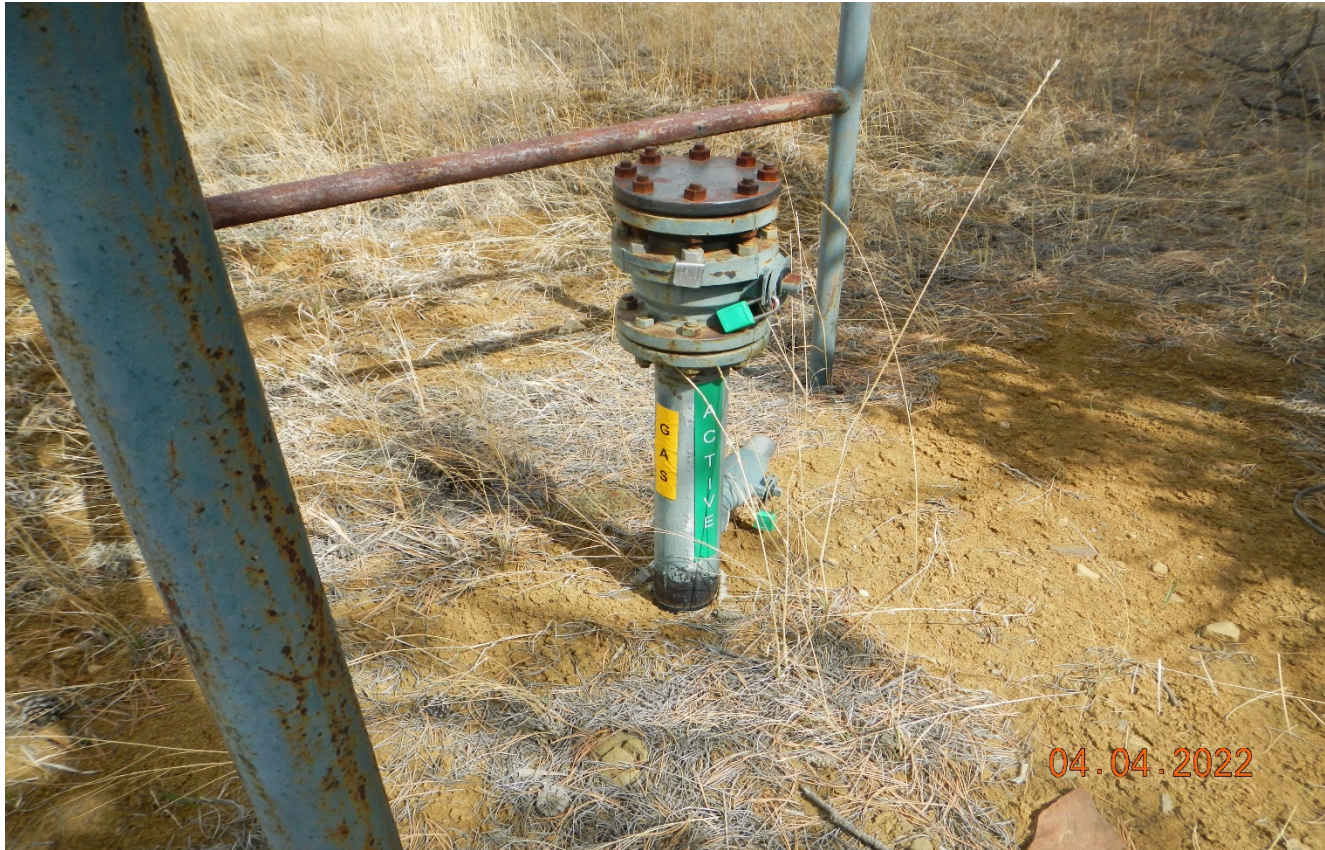
Photo 2. The pipe riser near the location and adjacent to the main road is LO and labeled as active line.
