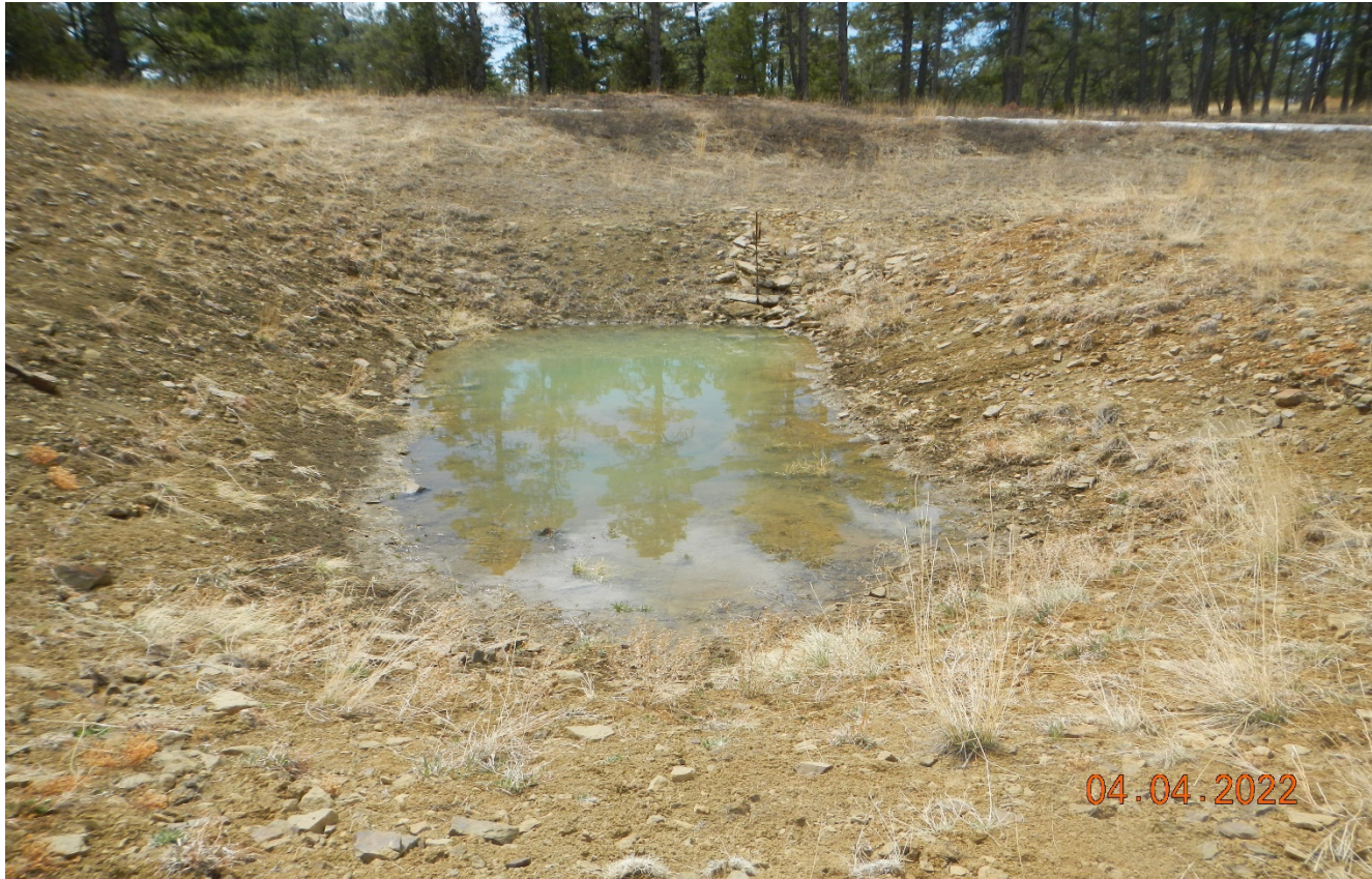
Photo 6. A shallow pit remains at the location and was never used for production. Pit remains per approved variance.
