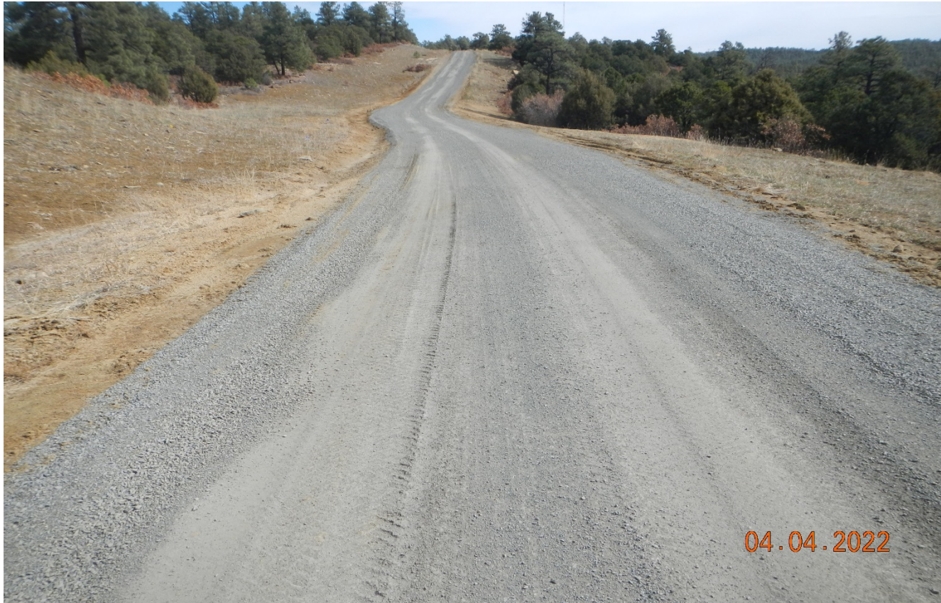
Photo 1. Facing northeast along the main road. Additional gravel has been applied to the road for stabilization.
