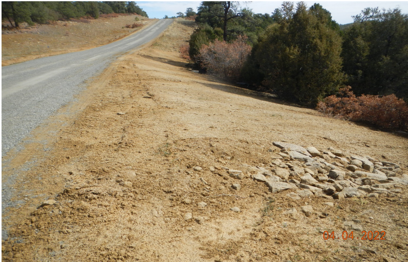
Photo 2. The area of erosion previously observed has been repaired, seeded, and stabilized.
