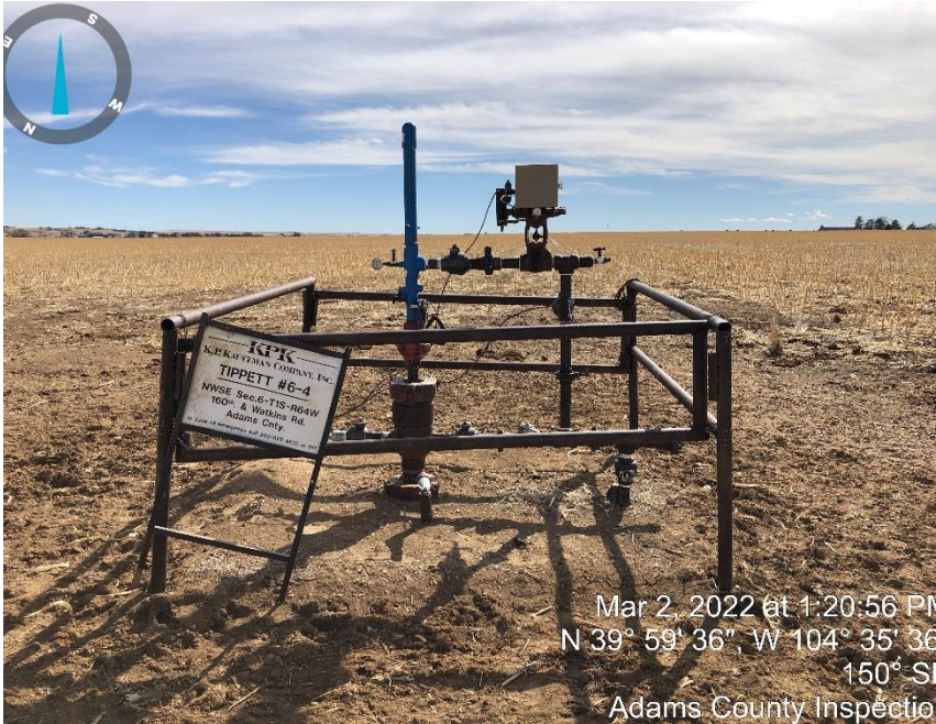
Photo #3 Well Head.
