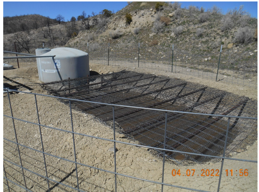
Blowdown tank and pit with fence/net
