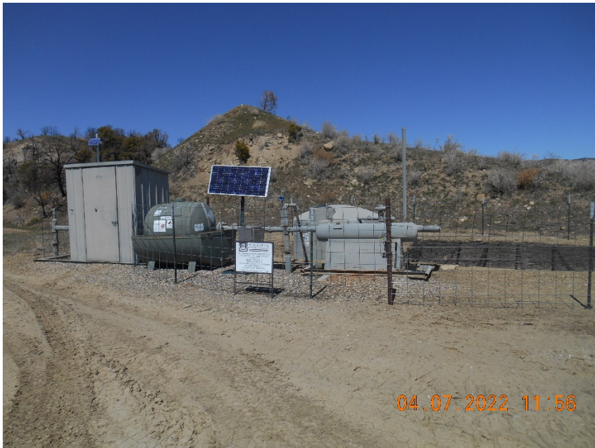
Separator and Meter housing
