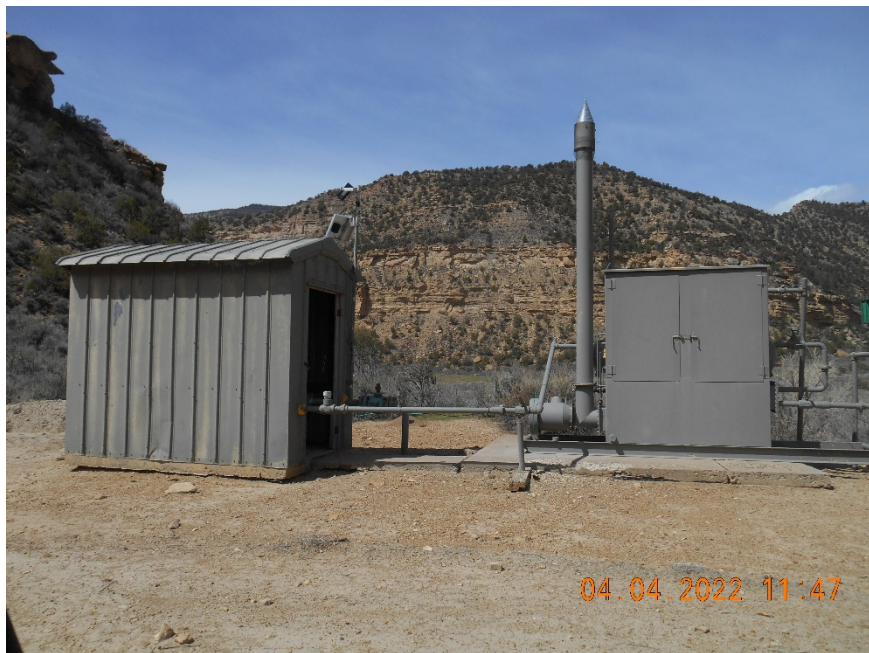
Separator and Meter housing.
