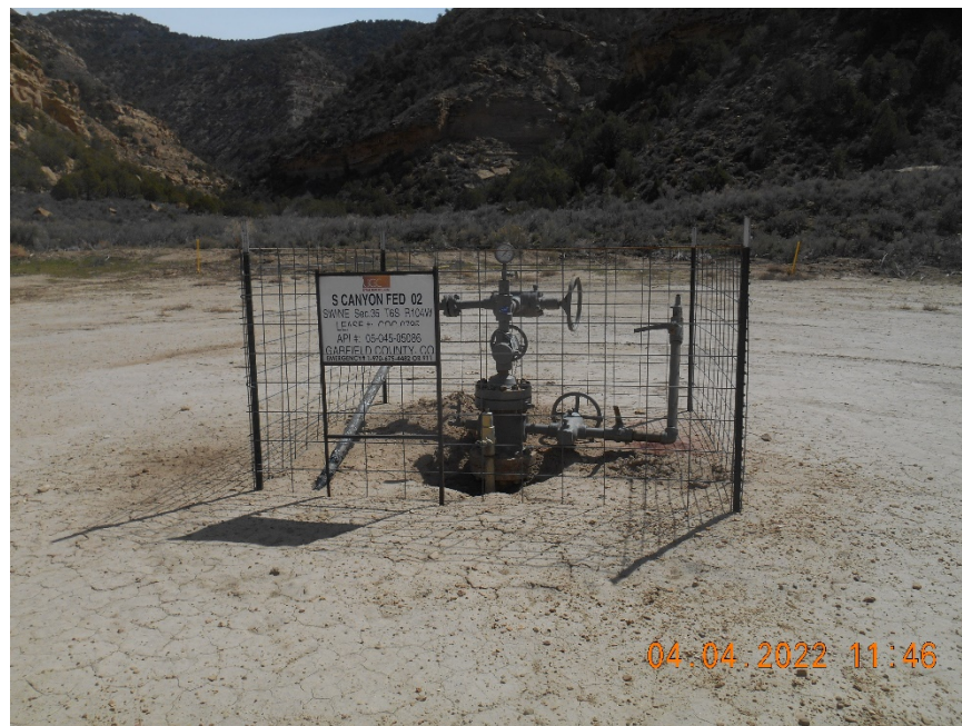
Wellhead with fence and sign.
