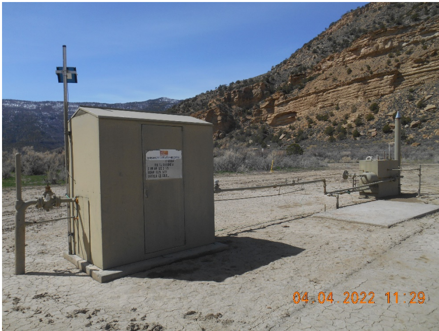
Separator and Meter Housing
