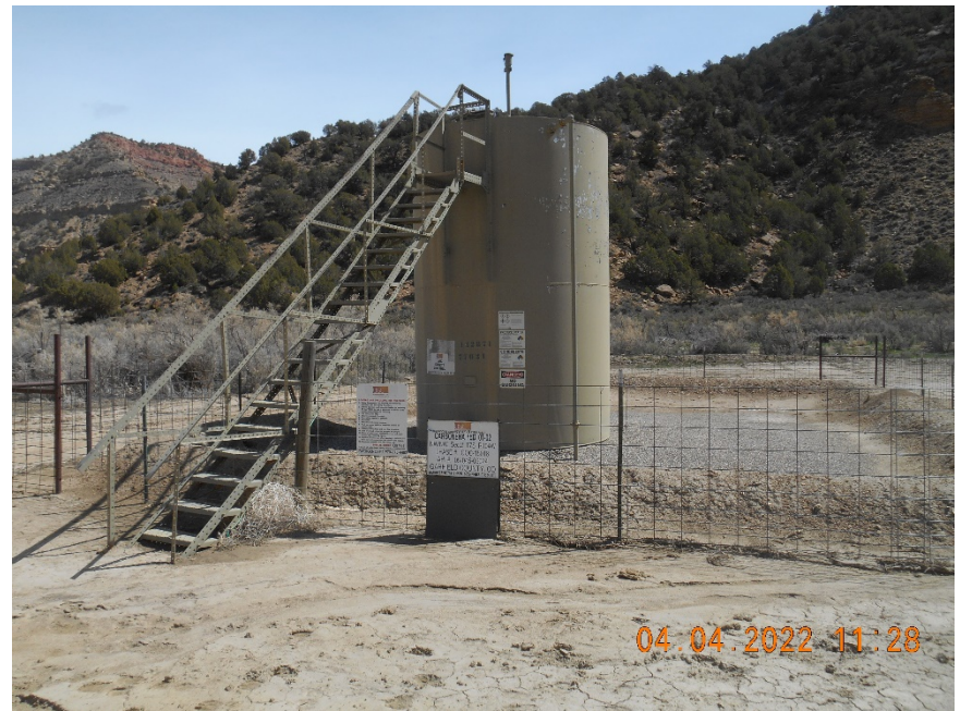
Tank battery with sign
