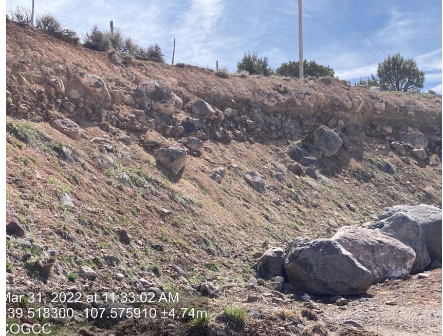
Lack of stabilization/compaction/erosion
