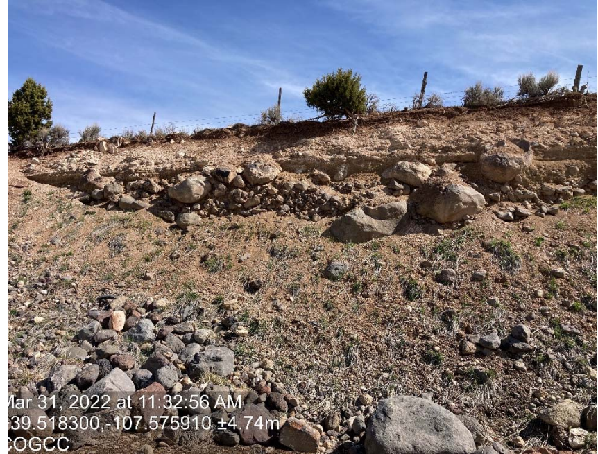
Lack of stabilization/compaction/erosion
