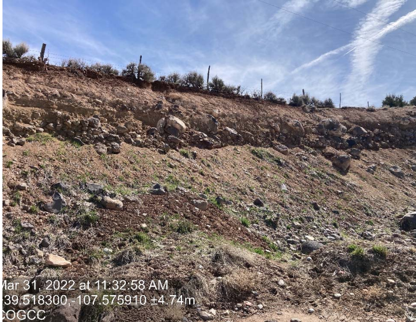
Lack of stabilization/compaction/erosion
