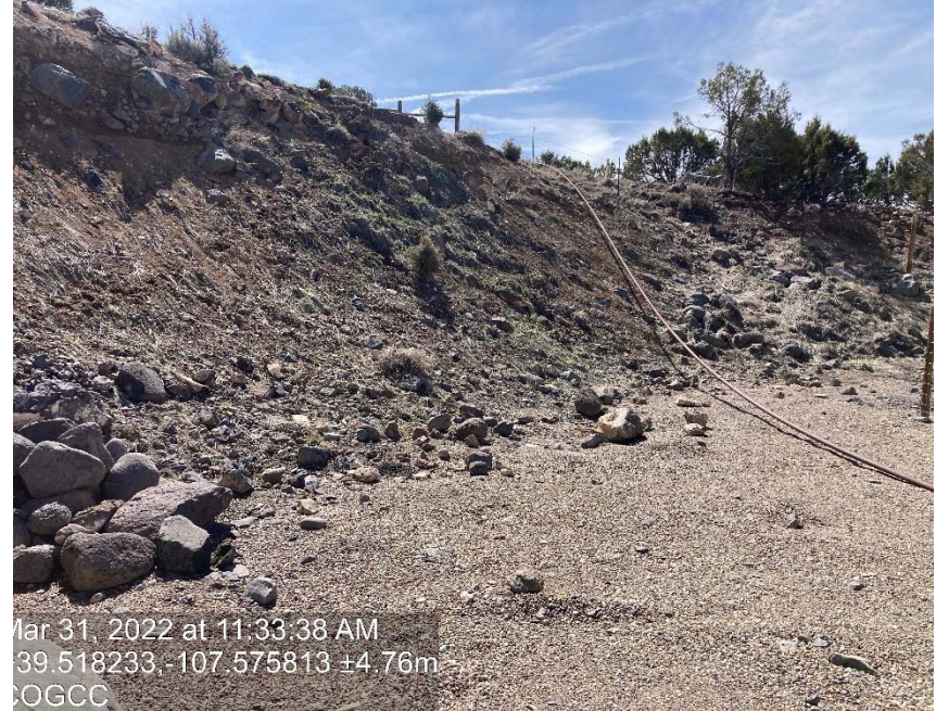
Lack of stabilization/compaction/erosion
