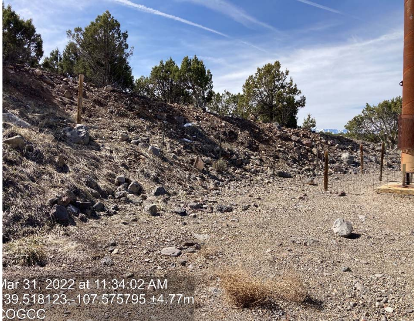
Lack of stabilization/compaction/erosion
