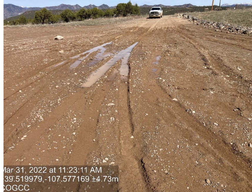
Lack of stabilization/compaction
