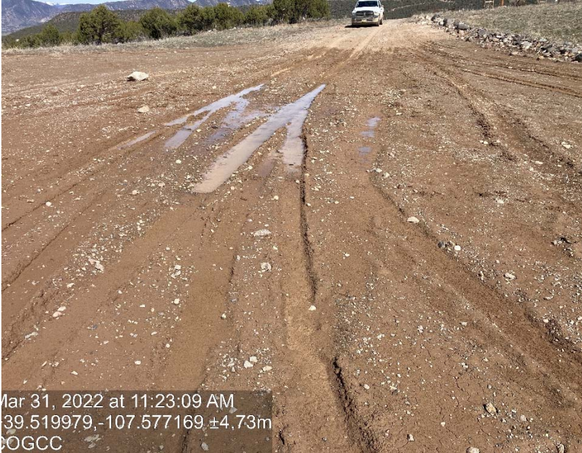
Lack of stabilization/compaction
