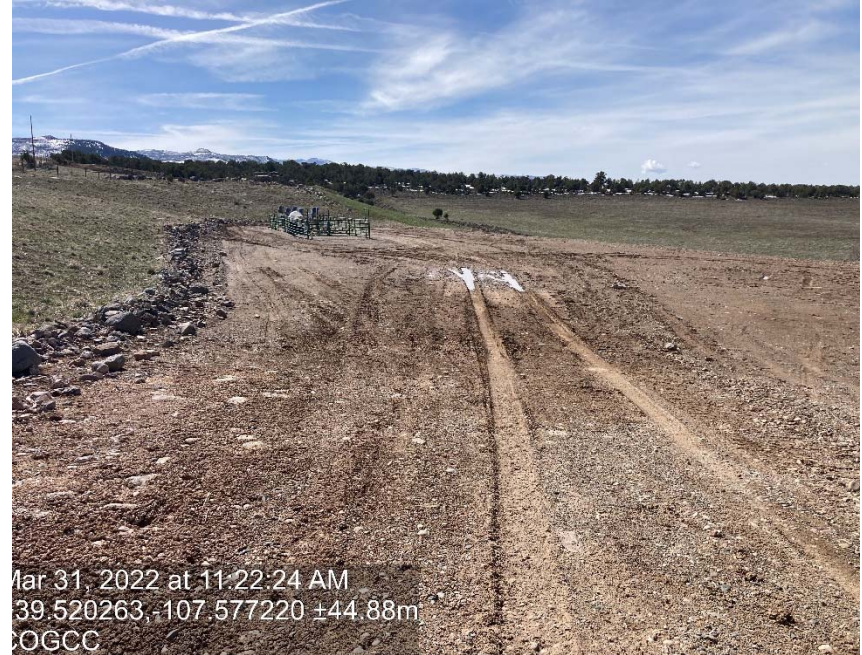
location/ Lack of stabilization/compaction
