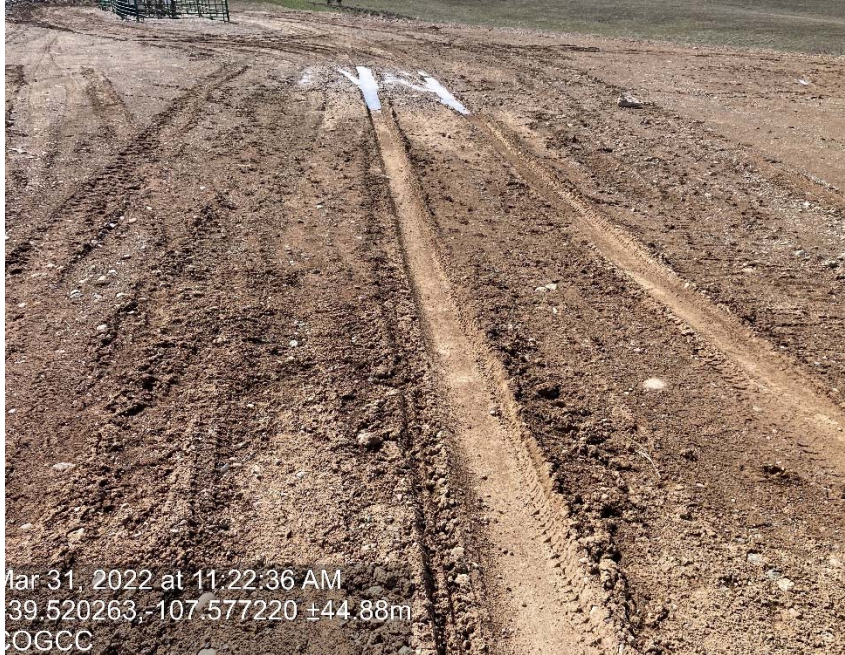
Lack of stabilization/compaction
