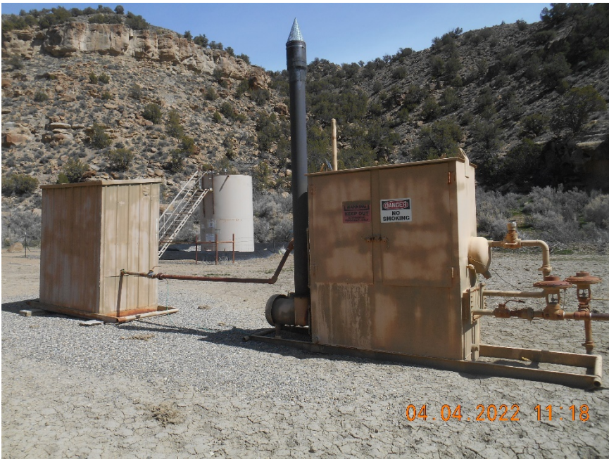
Separator and Meter housing.
