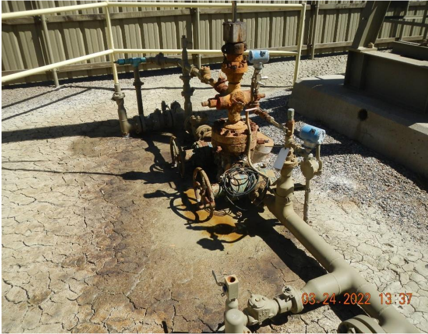
Standing water beneath #17-3 well head.
