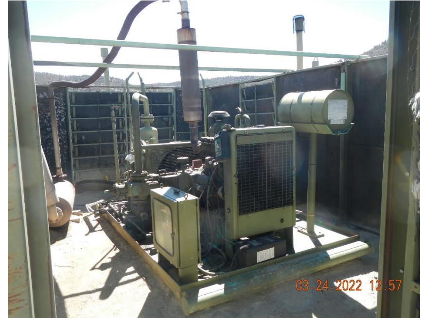
Compressor within sound walls.
