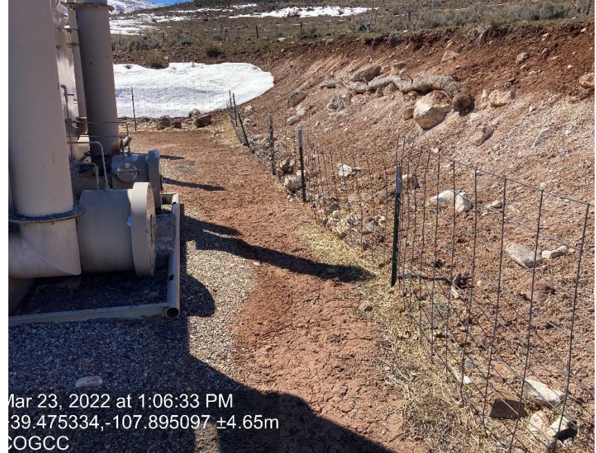
Lack of stabilization/compaction/erosion
