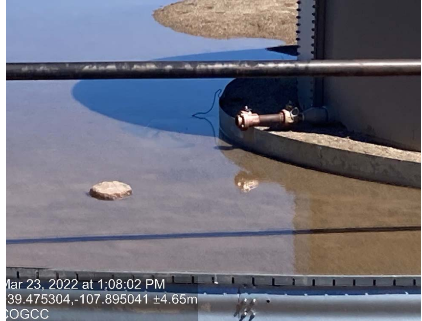
Valve missing cap/plug
