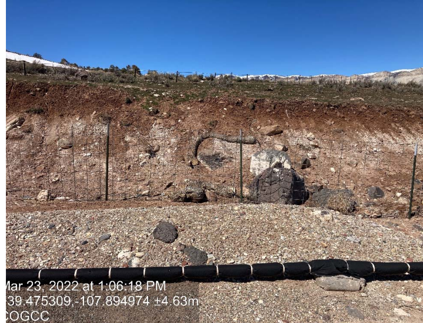
Lack of stabilization/compaction/erosion and debris
