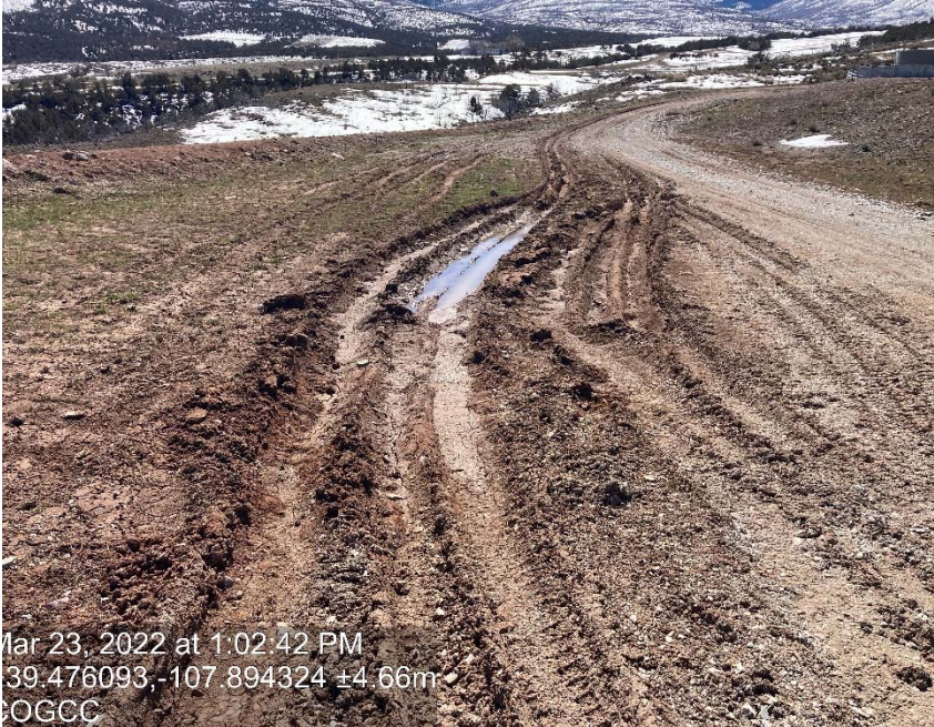
Lack of stabilization/compaction
