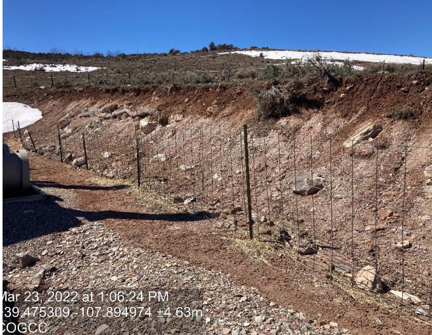
Lack of stabilization/compaction/erosion
