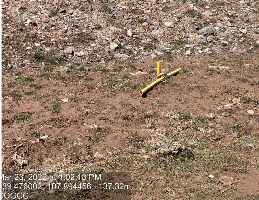
Dead men not marked properly
