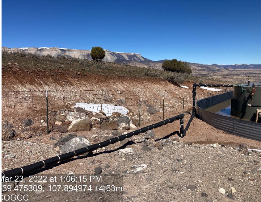
Lack of stabilization/compaction/erosion
