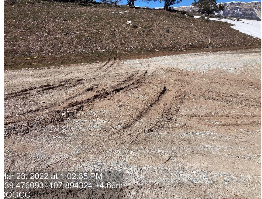
Lack of stabilization/compaction
