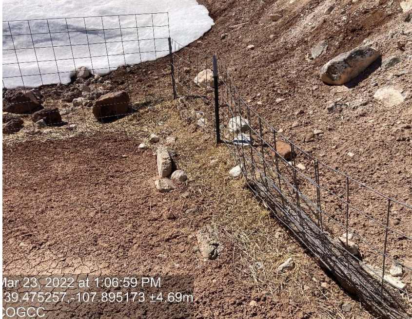
Lack of stabilization/compaction/erosion
