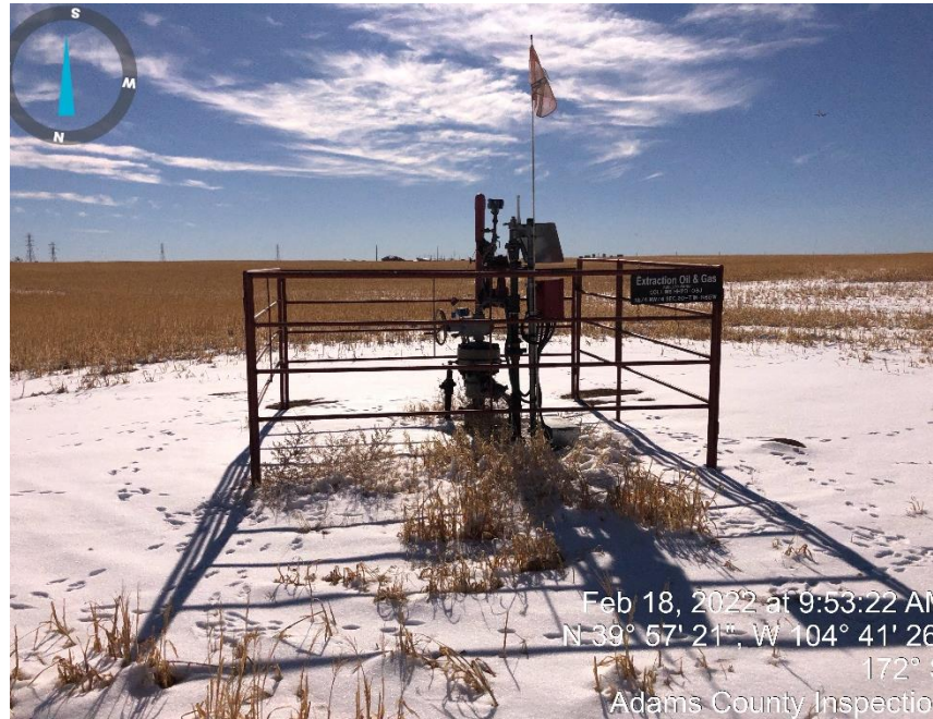
Photo #3 Well Head.
