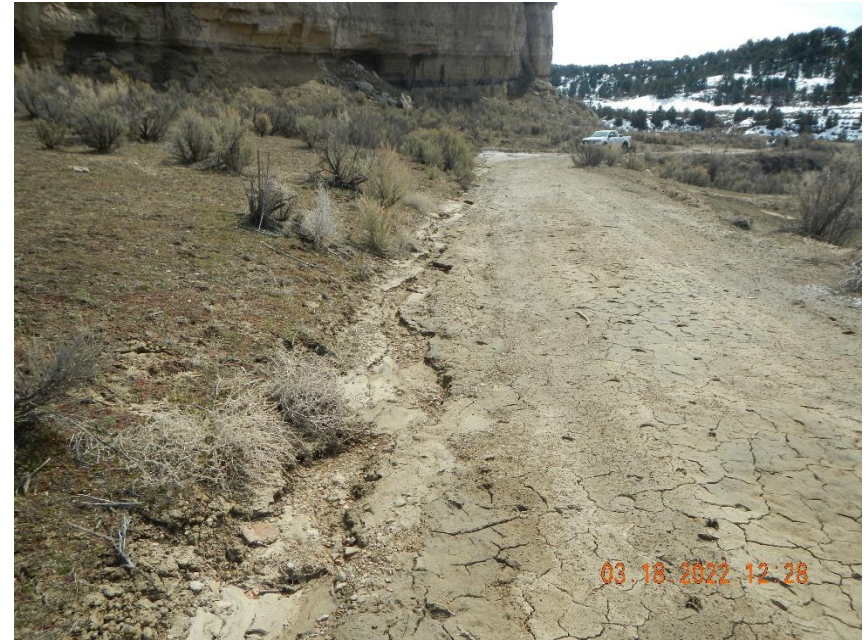
Ditch on main road needs maintained.
