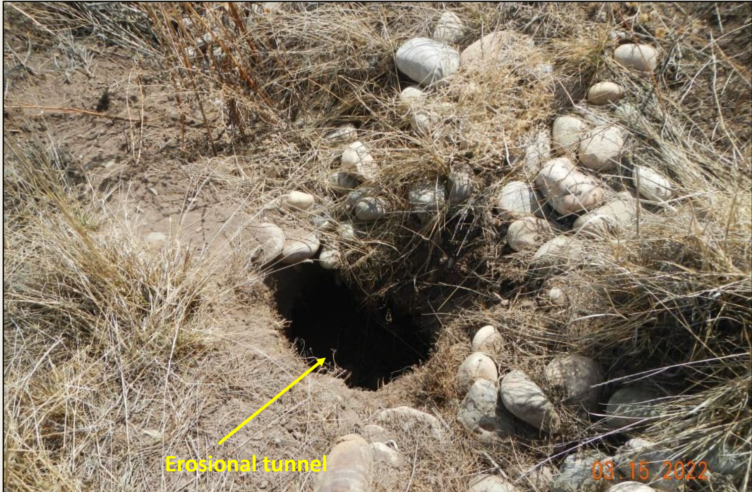
Photo 4. View of erosional tunneling in the southeastern corner of the well pad, approx. 2-3 ft deep. .
