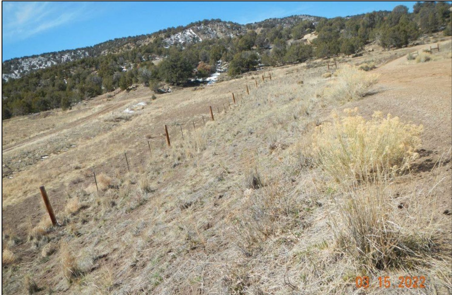
Photo 2. View of the southern fill slope from the southeastern corner facing westward. Revegetation is progressing with intermediate wheatgrass, crested whatgrass, and sand dropseed.
