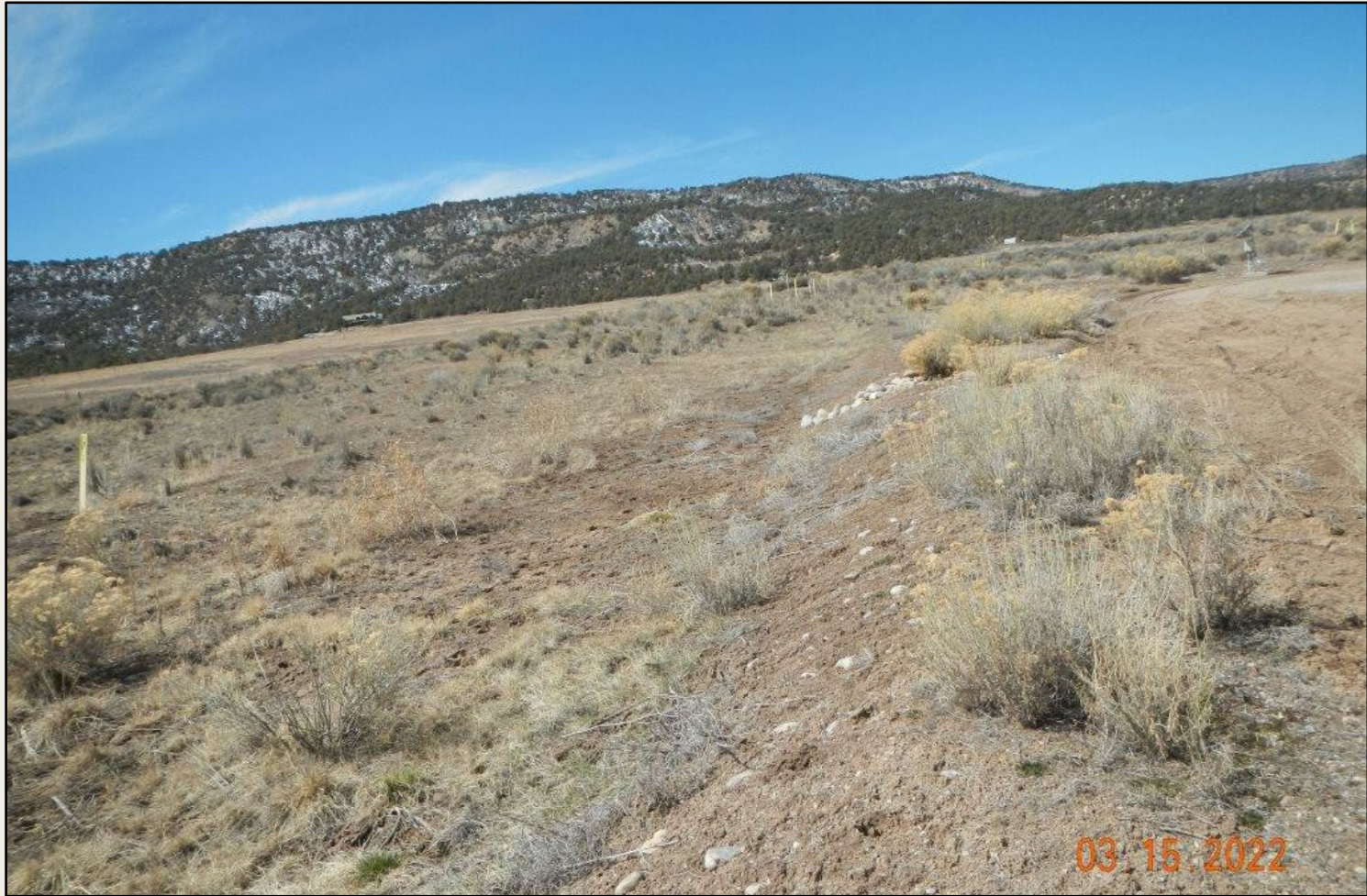
Photo 3. View of the southern fill slope from the southeastern corner facing westward.
