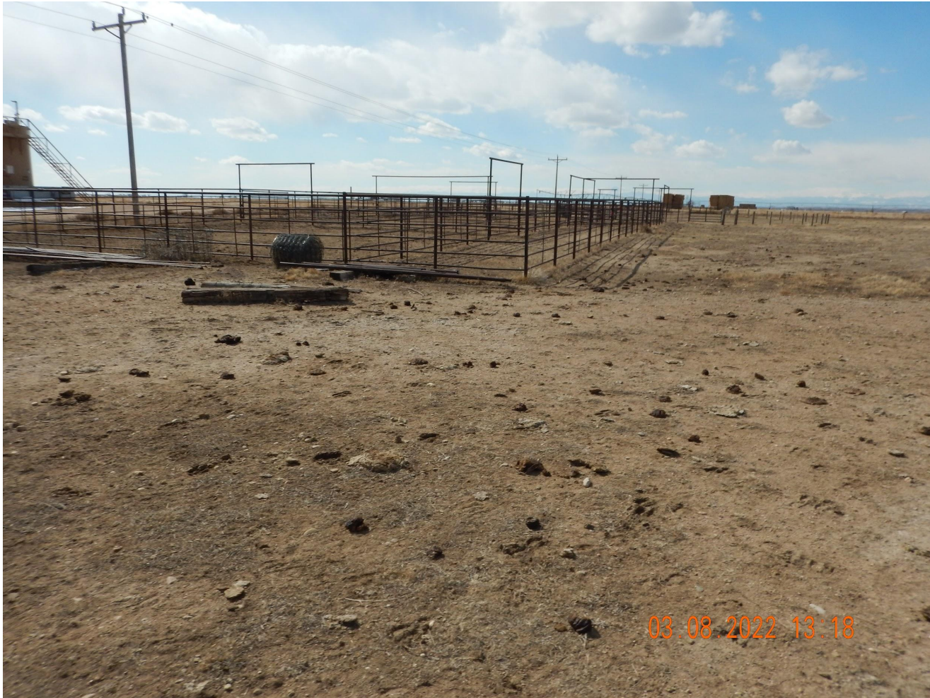
Photo 3. Photo taken from the associated tank battery, facing West. See comments under Photo 1.
