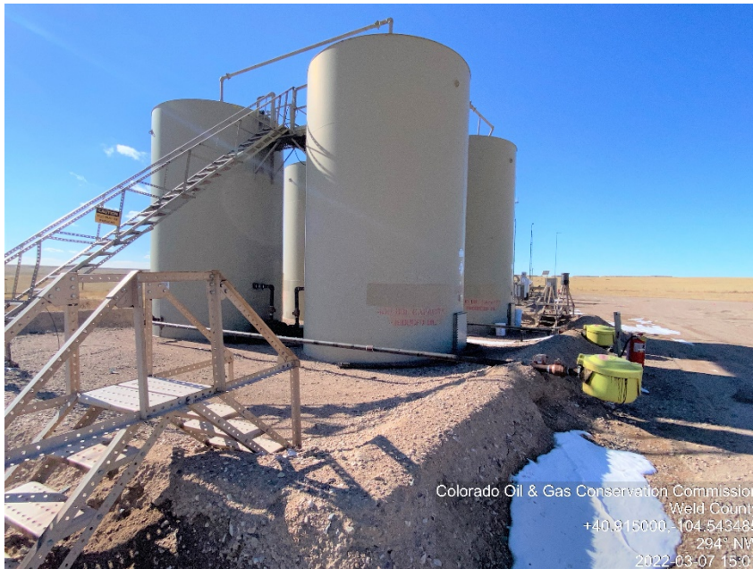
Photo #3 Lion Creek 4-16H Battery site Active Tanks, SE corner
