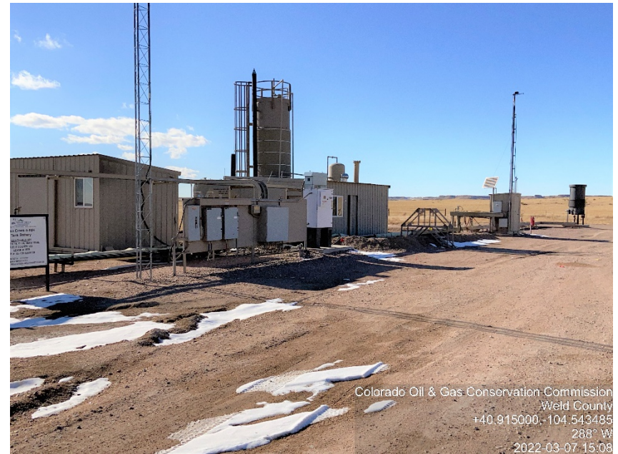
Photo #4 Lion Creek 4-16H Battery site Active Treater, Separator, Compressor, ECD
