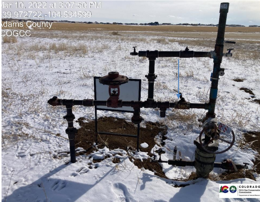
Pic 1 wellhead, At time of inspection all valves were in close position except one valve that is seized slightly open valves downstream of seized valve are in close position.
