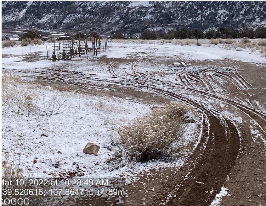
Location and Lack of stabilization/compaction
