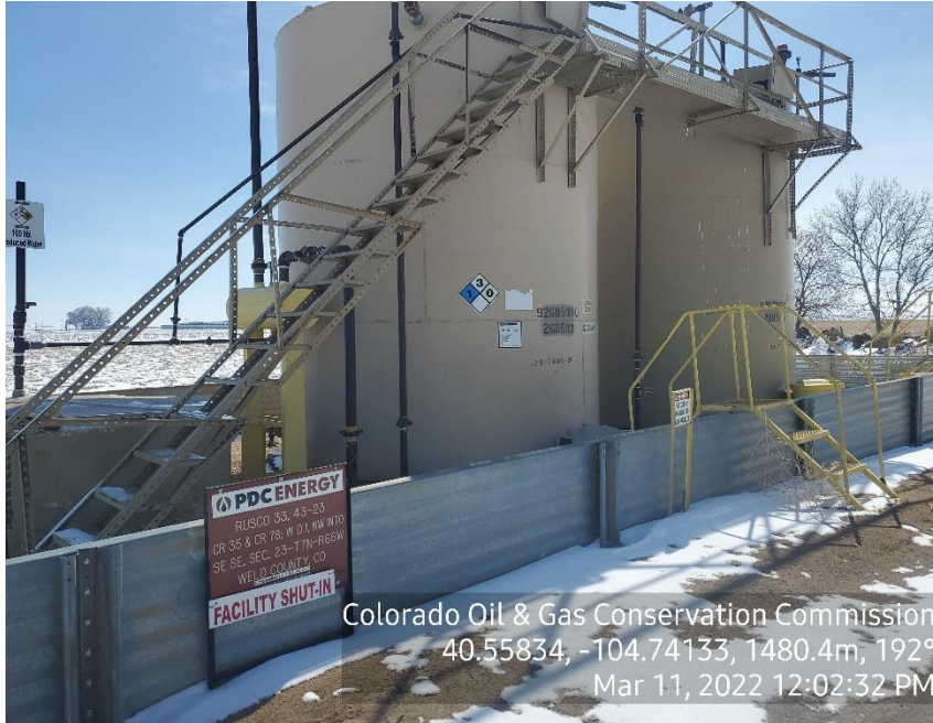
Photo 3: Centralized Tank Battery
