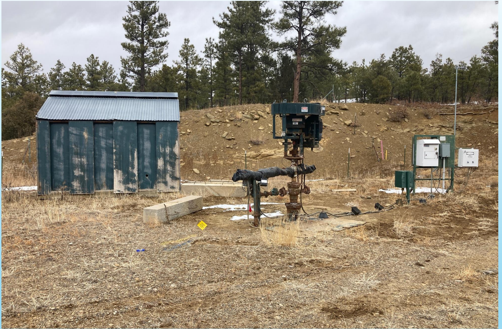
PHOTO 3: WELL EQUIPMENT/ UNUSED EQUIPMENT (CONCRETE SKID CHOLKS & SOUND WALL CHED). REMOVE UNUSED EQUIPMENT, COMPLY WITH RULE 606. CA DATE 3-21-2022.
