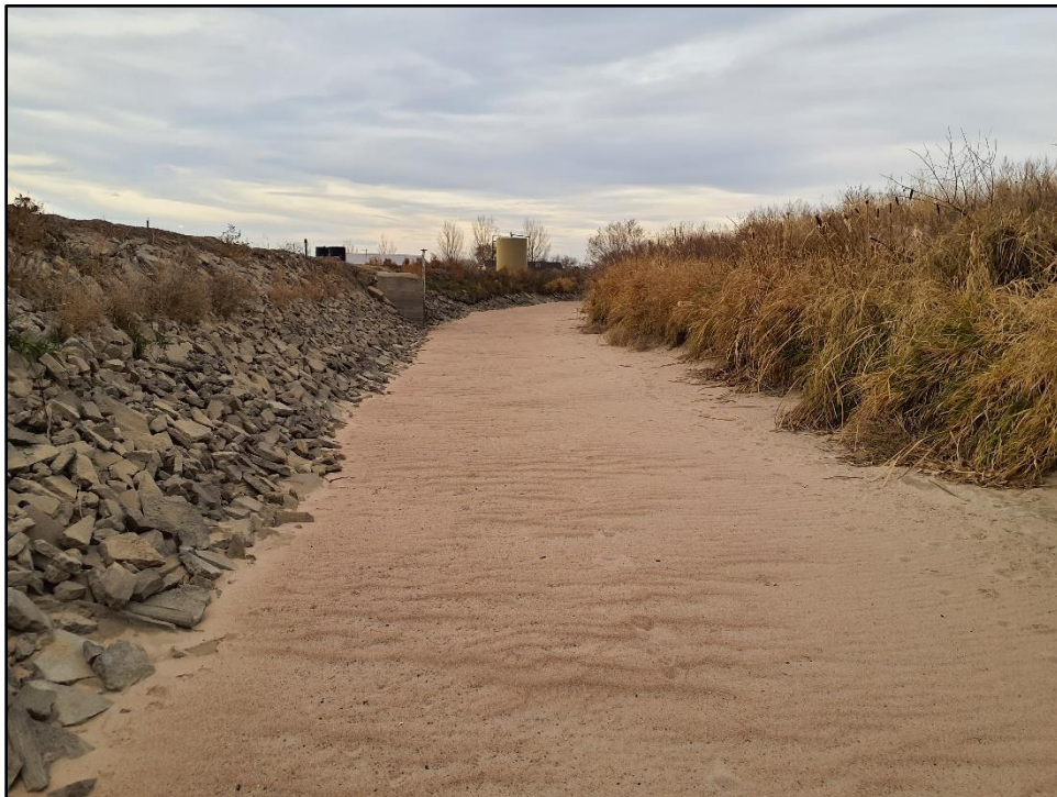
Figure B5. Overview of Greely Number 2 Canal in A07-04 survey area, facing west.
