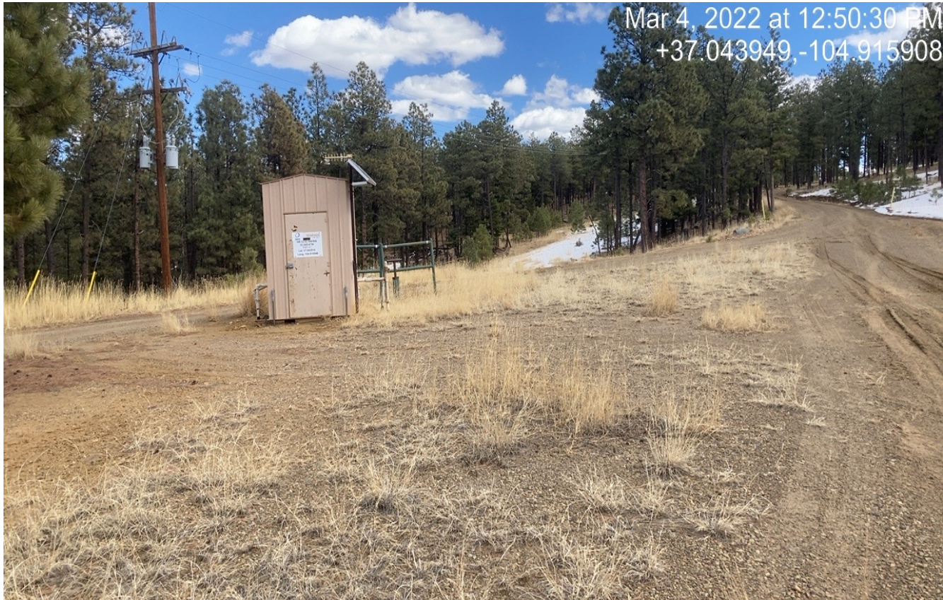
Photo 2. Well sign is posted at meter shed.
