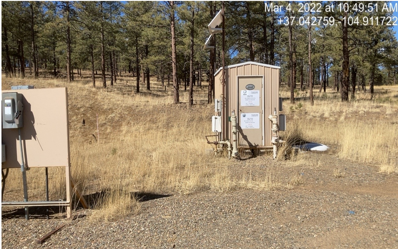
Photo 3. Well sign posted at meter shed.
