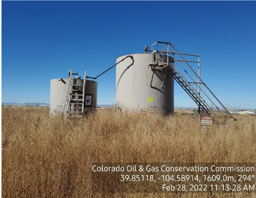
Photo 3: Centralized Tank Battery
