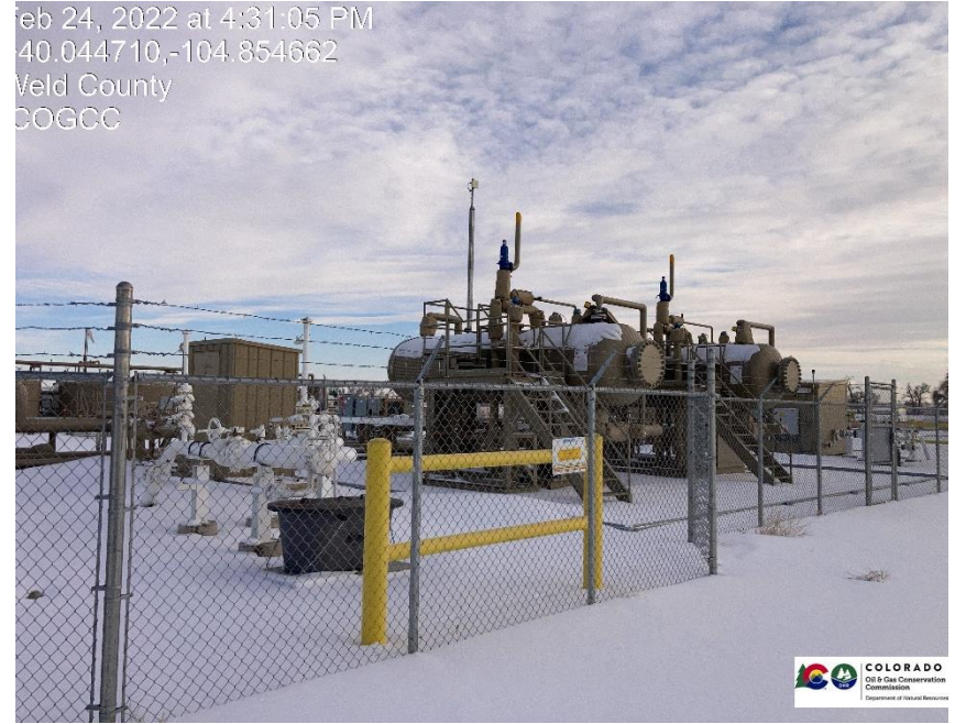
Pic 4 Gas meter run, separators, LACT
