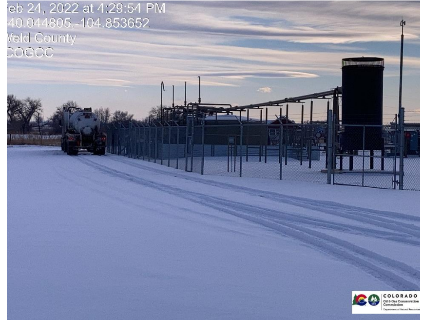
Pic 2 tanks, ECD
