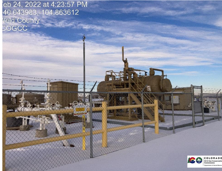
Pic 3 Gas meter run, Separator, LACT
