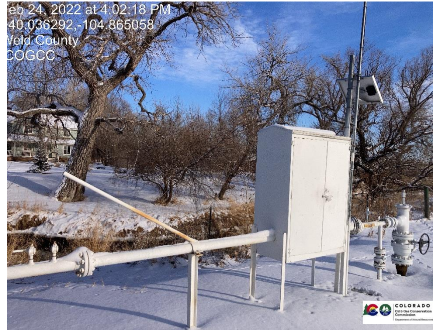
Pic 2 gas meter run
