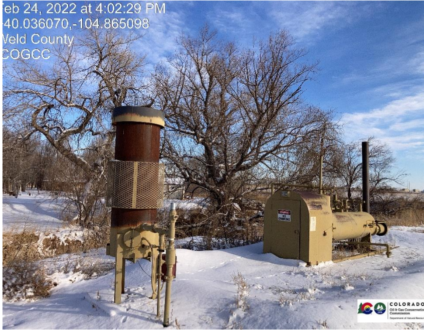
Pic 3 ECD, separator
