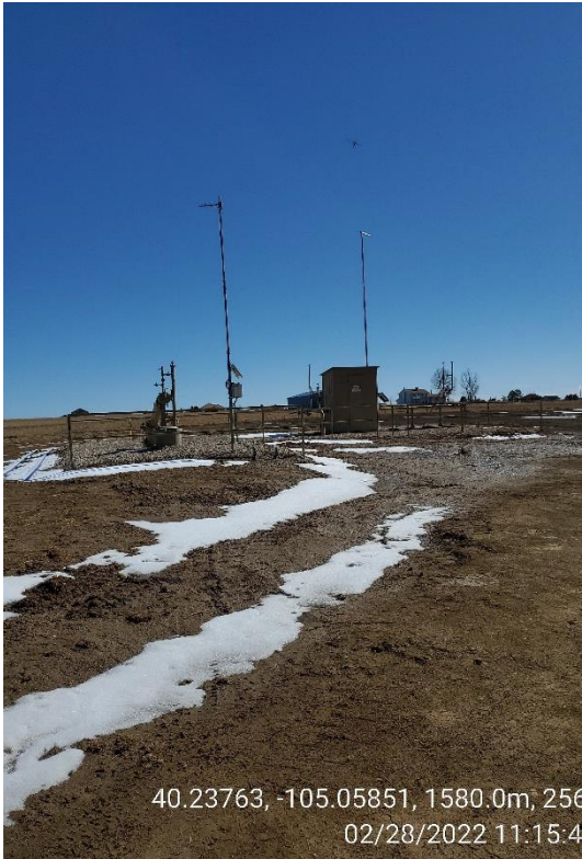
Photo 1 GMR and Pig Station
