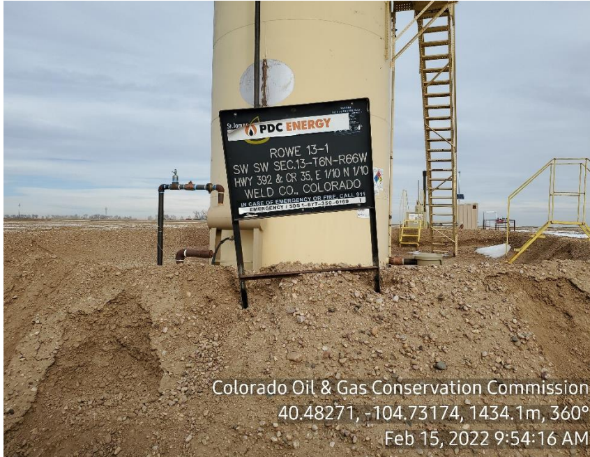
Photo 1: Tank Battery Sign
