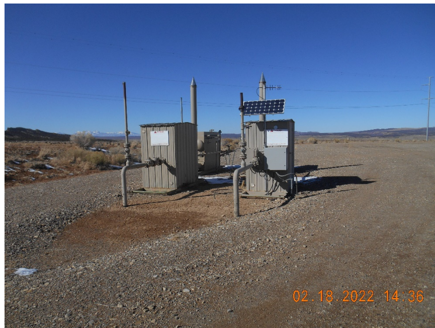
Separators and Meter housings
