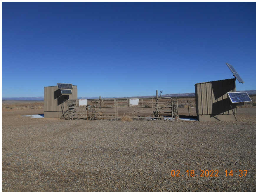
Wellheads with fence and signs
