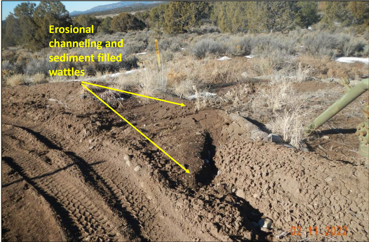
Photo 3. View of area in the northwestern project area where concentrated stormwater flows off of the working area. Erosional channeling and sedimentation observed on the working pad surface and flowing into wattles full of sediment and not longer functioning.
