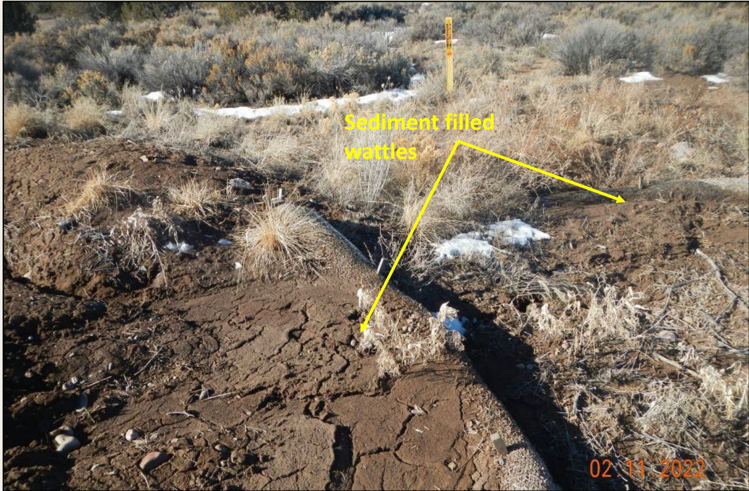
Photo 4. View of sediment filled wattles in the northwestern project area, downstream from Photo 3.
