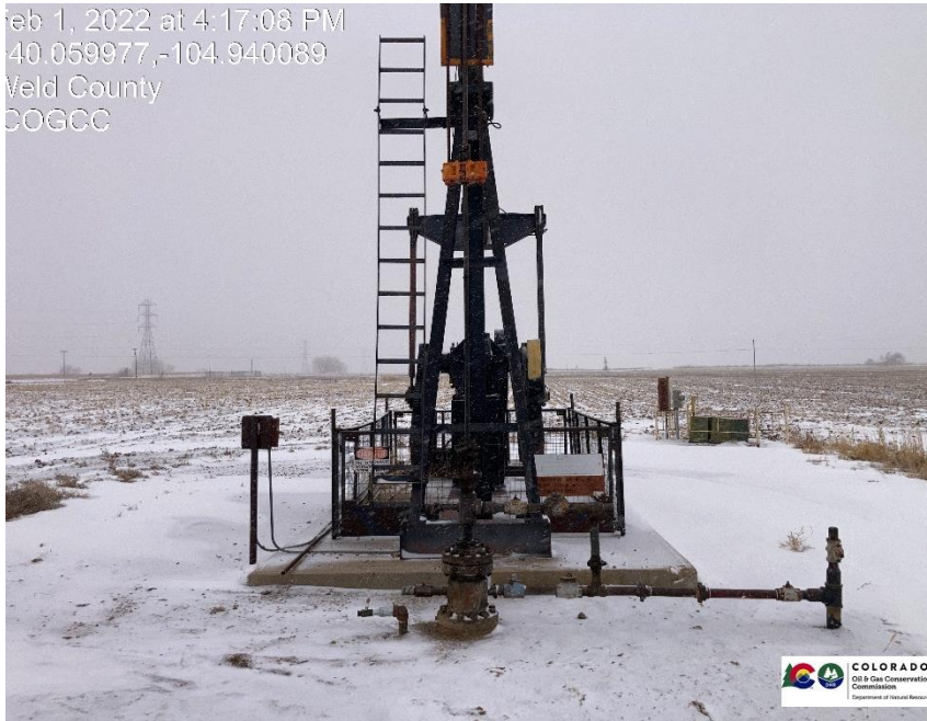
Pic 2 wellhead, electric equipment, pump jack
