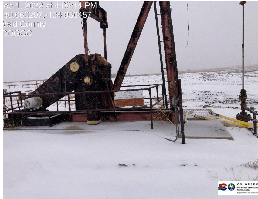
Pic 1 wellhead, pump jack.
