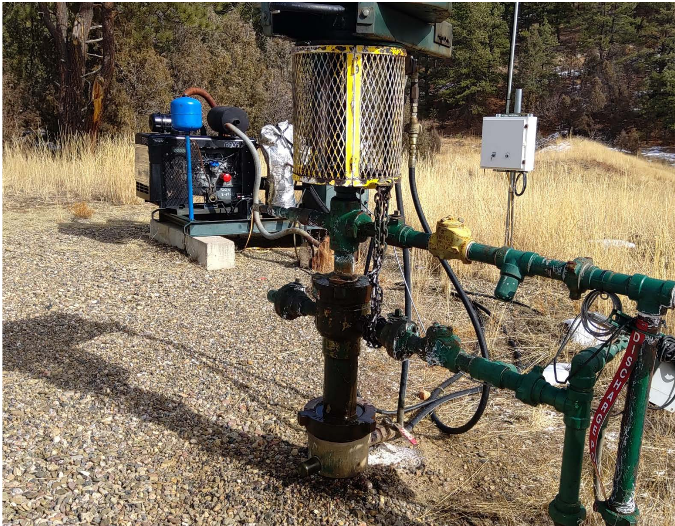
TR well where leak was observed.
