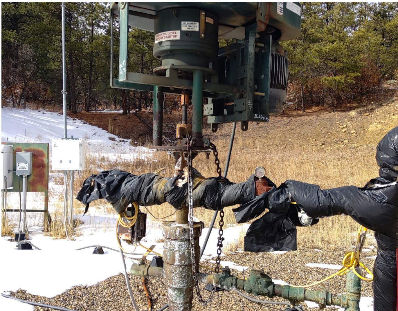
Boxster 12-13 well. Salt buildup on wellhead indicate previous leak from wellhead.
