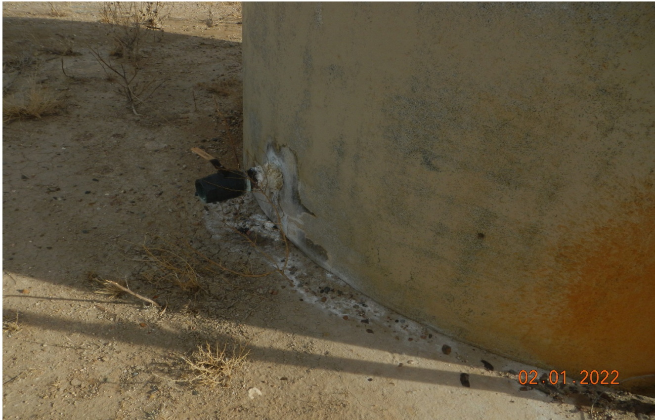
Photo 9. There are signs of a previous leak at the pipe fitting.
