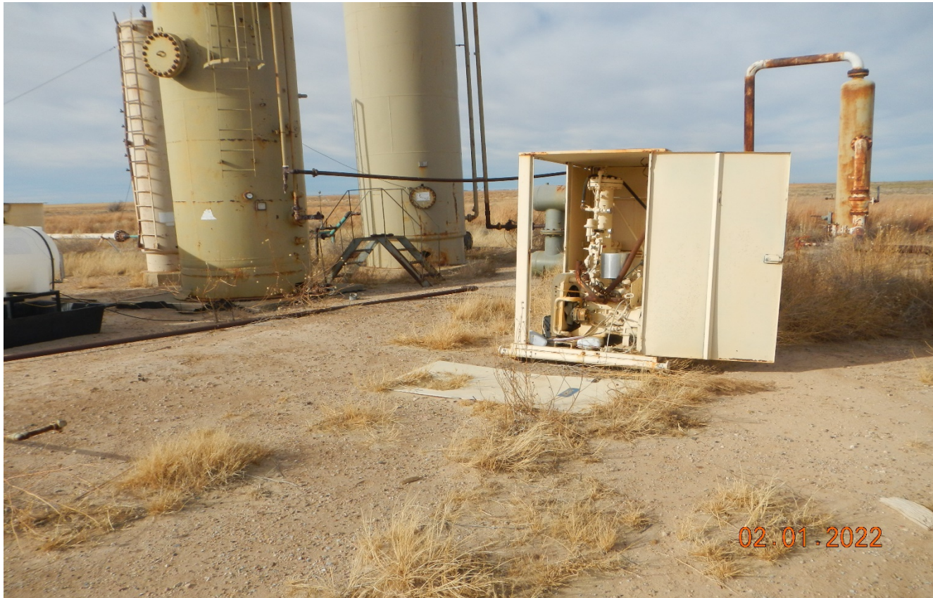
Photo 6. There is unused or equipment not maintained on location. Door has fallen off this shed.
