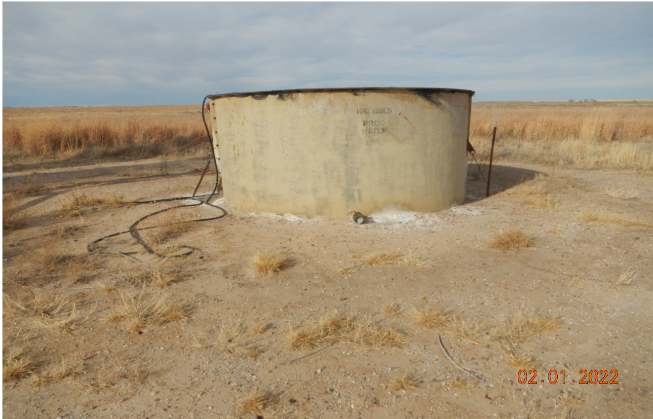
Photo 7. There is an open top tank at the east side of the location. It appears the tank has previously leaked due to white stained soil. There is no secondary containment around the tank. The signage has faded.
