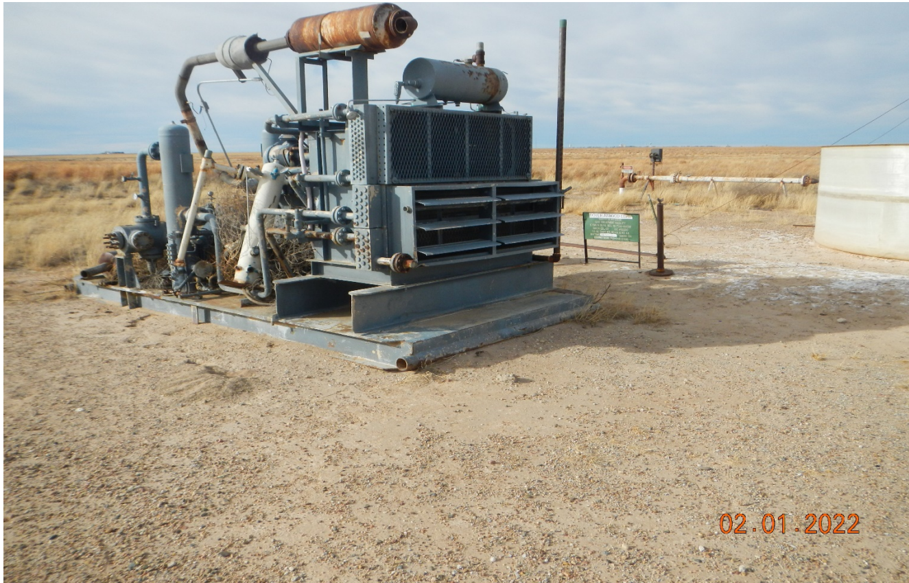
Photo 2. There is an unused compressor stored on location that need to be removed.
