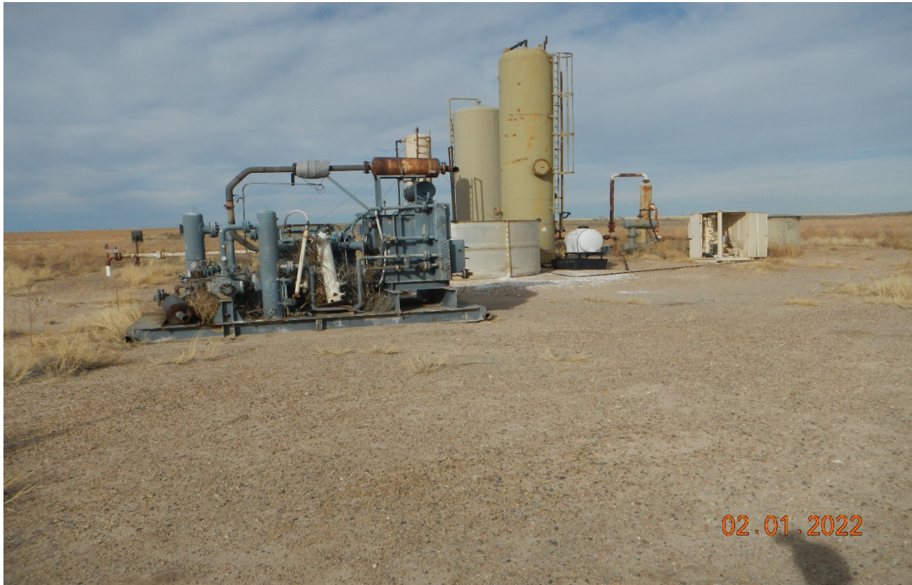
Photo 1. Facing northeast toward the gas treatment facility.
