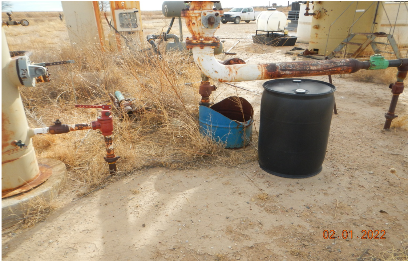
Photo 10. There is unused supplies and a black barrel with no labeling.
