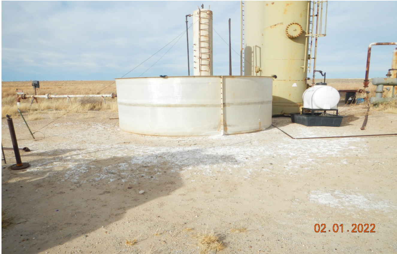
Photo 4. Facing toward the open top tank. It appears the tank has previously leaked due to white stained soil. There is no secondary containment around the tank. There is no signage on the tank.
