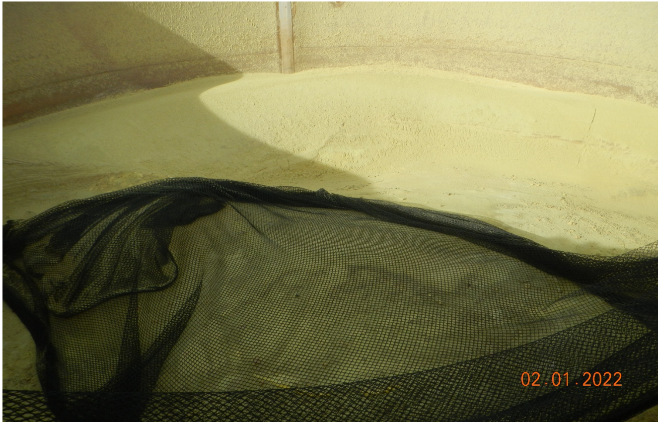
Photo 5. The netting over the tank is not installed.
